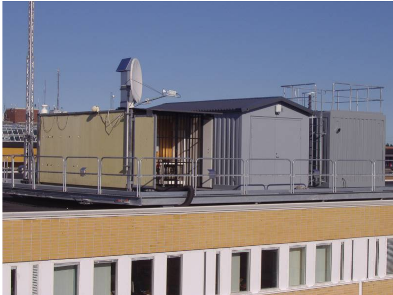
Fig. 3: The radionuclide measurement stations at FOI, Stockholm. The leftmost container holds the CTBT particulate station SEP63; the middle container is equipped with a CTBTO noble gas system (SEX63). The station to the right is a semi-automatic particulate sampler operated for the Swedish radiation authorities, and is not described in this report. The parabolic antenna to the left is the satellite link to the CTBTO International data Centre in Vienna.
